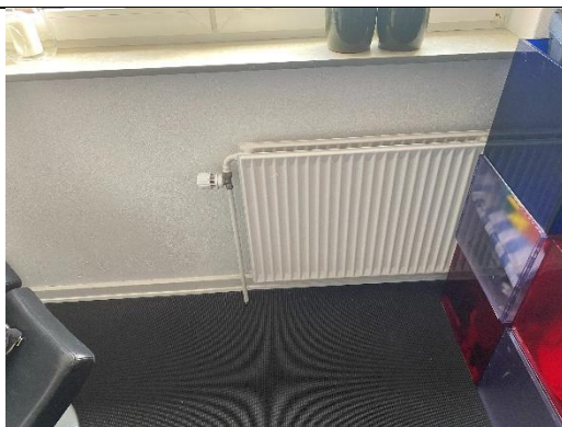
Radiator i stue
